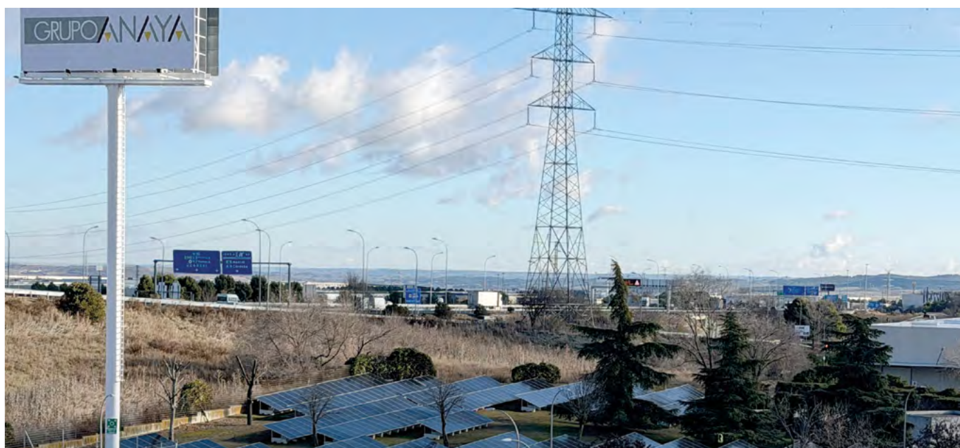
Installation of solar panels at the logistics site in Getafe, Spain (Grupo Anaya).
